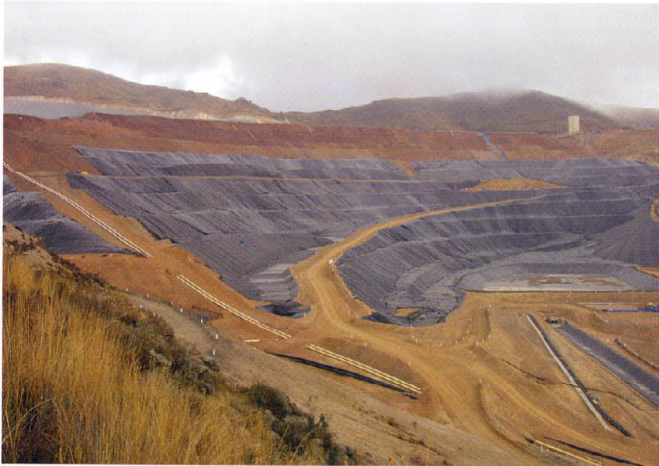
Photo 1 | Raincoat liners applied at the Pierina gold mine heap leach project located north of Lima, Peru. Rainwater is routed to a lined holding pond for reuse in mining operations.
