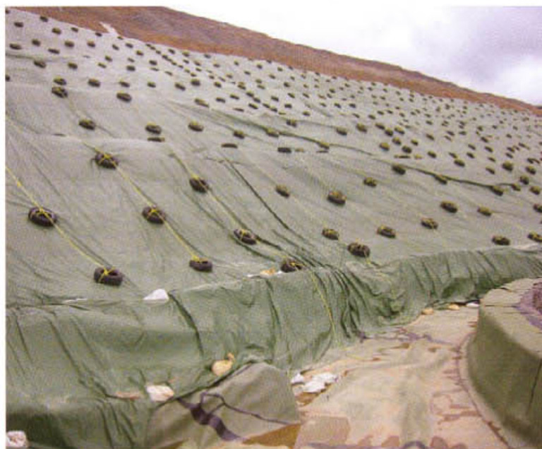
Photo 4 | In this example, the raincoat liner is anchored by tires and ropes for protection from the wind. Note the raincoat diversion channel in the foreground for diverting stormwater runoff to a lined pond for testing and release of storm freshwater flows.
