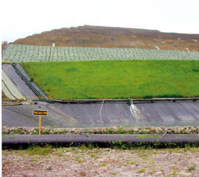
Photo 3 | Raincoat liner cover startup installation on bottom slopes of a gold heap leach pad in Costa Rica. Stormwater runoff is diverted to the lined pond shown in the foreground for water-quality testing and release to natural drainages.
